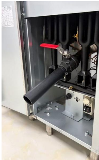
Figure D – Drain extension installed on drain valve
